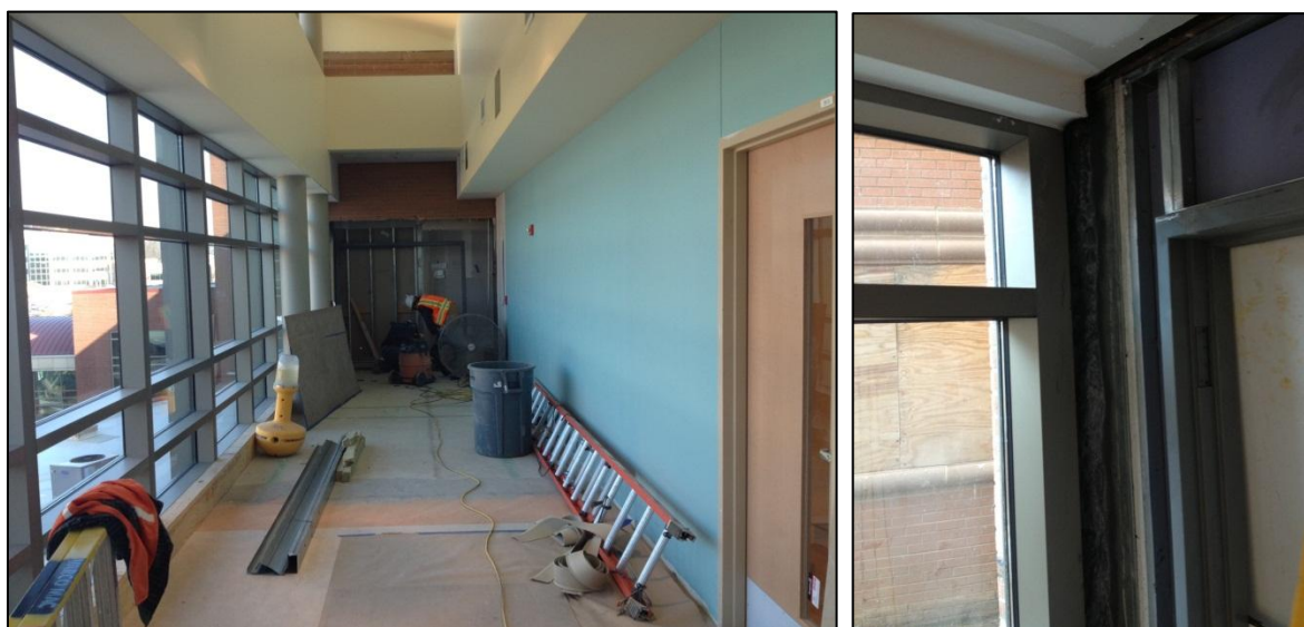
Figure 57, Left - Laborers working on the expansion joint between the floor slabs of the existing floor slab and addition. Issues required this scope of work to take much longer than anticipated due to the slabs not lining up as intended. Right - Building connection between the addition's aluminum curtain wall and existing building. Framing and a door frame can be seen already in place.
