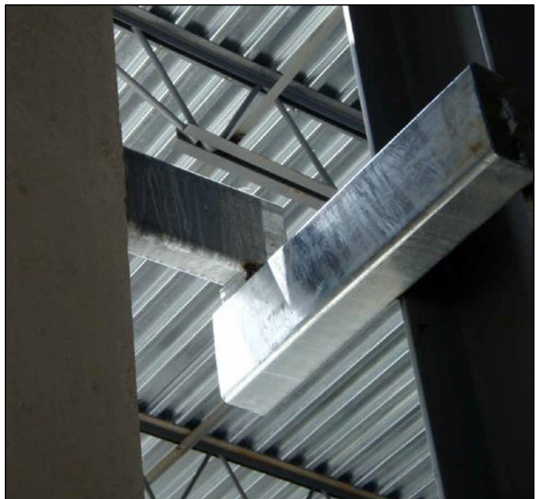
Figure 31 - Photo of a similar connection supporting a precast panel. Shims can be seen between the tub steel used, similarly to the left section, to prevent thermal bridging. Image from the NCPA Architectural Precast Connection Guide.
