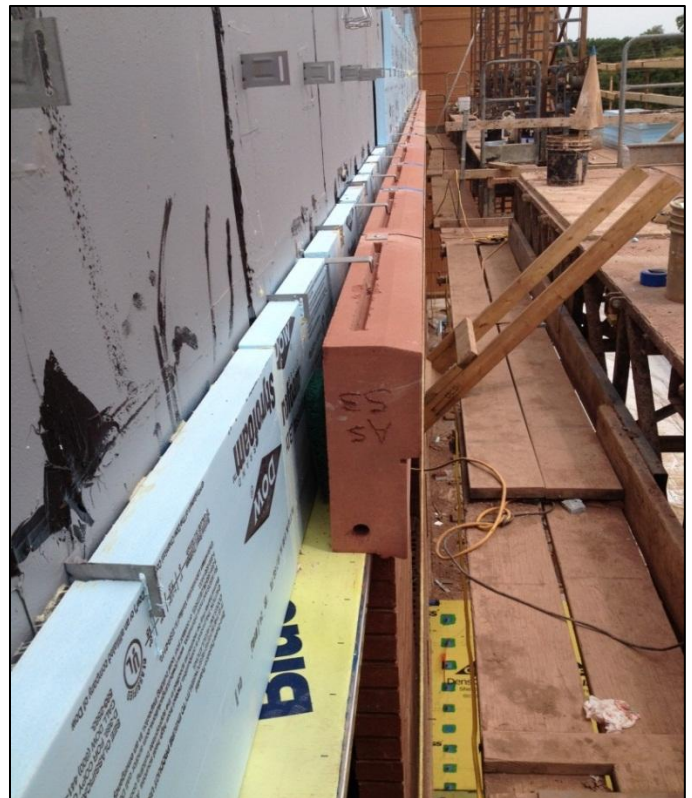
Figure 10 - Precast concrete can be seen above which make up the accent band along with east elevation. Personal photograph taken by Chris Pozza.
