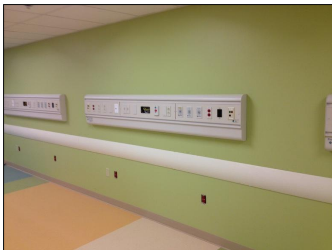
Figure 62 - Modular headwall units used on the project. This image was taken on the third floor of the KP Medical Office Building. Personal photograph taken by Chris Pozza.
