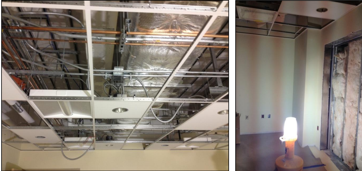
Figure 25 - Images of the CT Imaging room ceiling and temporary light fixture used inside the space. This picture was taken after a ceiling close-in inspection was performed and approved. An issue with the lead-lining required all utilities and the ceiling overhead in this room to be removed. Personal photographs taken by Chris Pozza.
