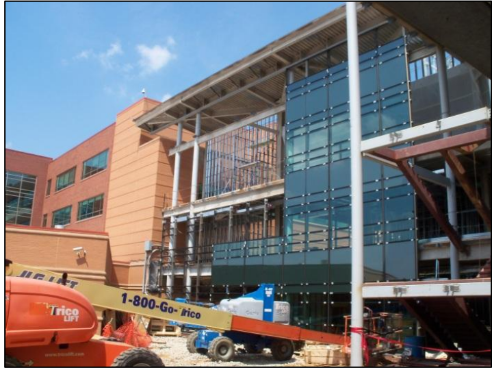
Figure 16 - View of west elevation curtain wall system under construction. The boom lift used during construction of the façade system can be seen at the bottom of the photo. Personal photograph taken by Chris Pozza.
