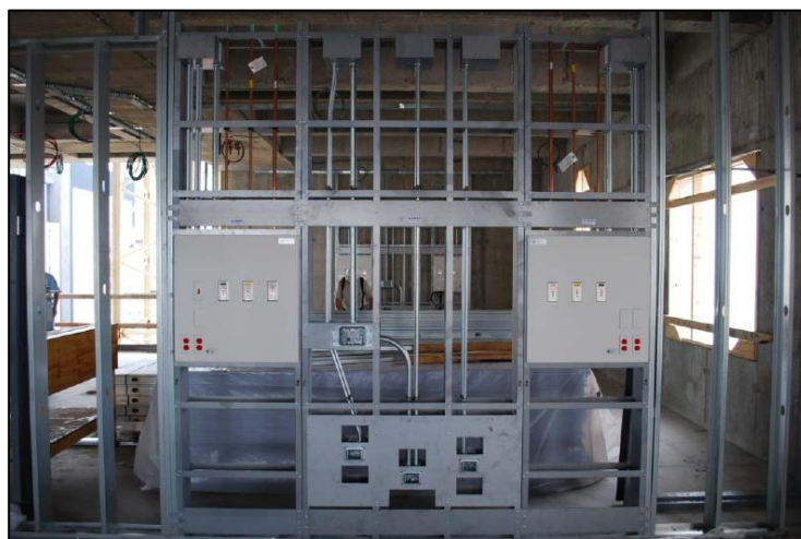
Figure 63 - Proposed headwall module. The entire unit consists of piping, conduit, wiring, framing, and other necessary components. Connections are made above the finished ceiling for a convenient means of installation as no vertical drops are necessary to be roughed in. Image from Modular Services.
